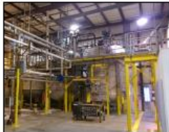
Wet (Reactor) Processing
